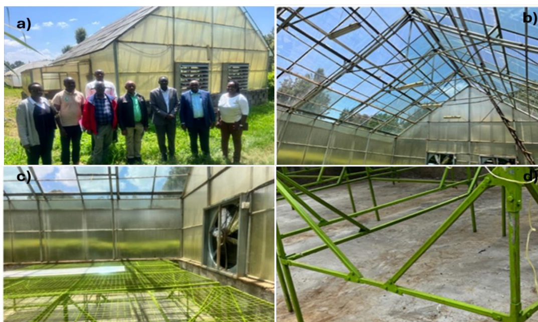
Figure 2. EGU BREEDTECH Center 2 at Egerton University, Kenya. (a) The glasshouse status during site handover to the contractor; (b) Replaced glass panes; (c) Refurbished benches and (d) Concrete floor
