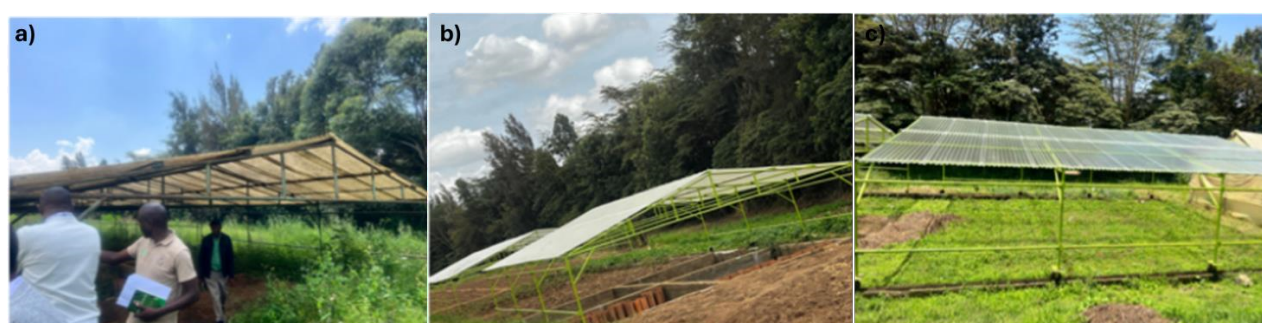
Figure 1. EGU BREEDTECH Center 1 at Egerton University, Kenya. (a) Old rain shelter before rehabilitation and (b)& (c) rehabilitated rain shelter. The upgrades included re-roofing, restoration of wheel rails, and painting
